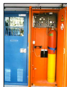
Figure 3: Gas Cylinder Cabinet
