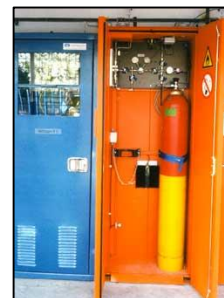
Figure 3: Gas Cylinder Cabinet
