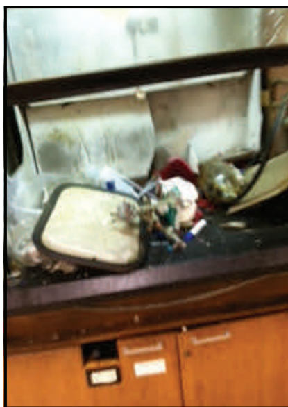
Fig. 1 TX Tech, damaged fume hood.
