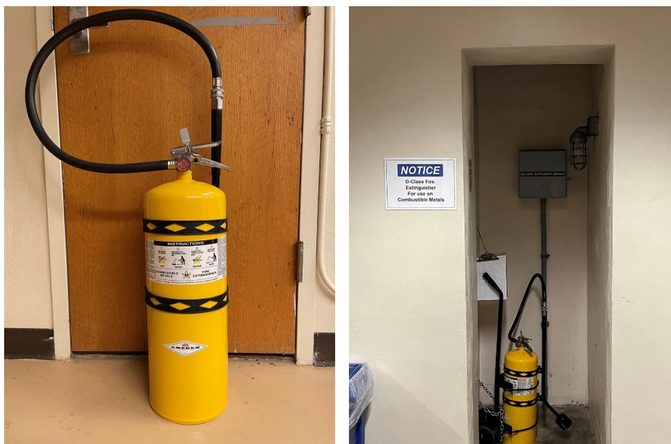
Class D Fire Extinguisher (CDFE), located between WTHR 419 and 420 (locked)
